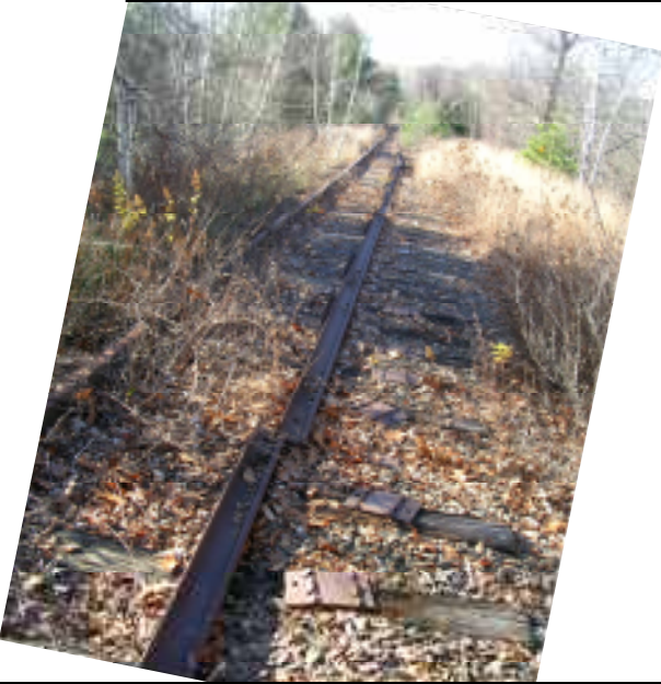
Looking west along at the loose tracks left behind by the salvage crew in 1994. The embankment is above Longacre Landscaping
